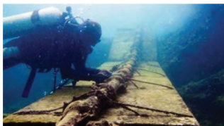
Underwater Internet Cable Infrastructure
